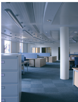
Active chilled beams
