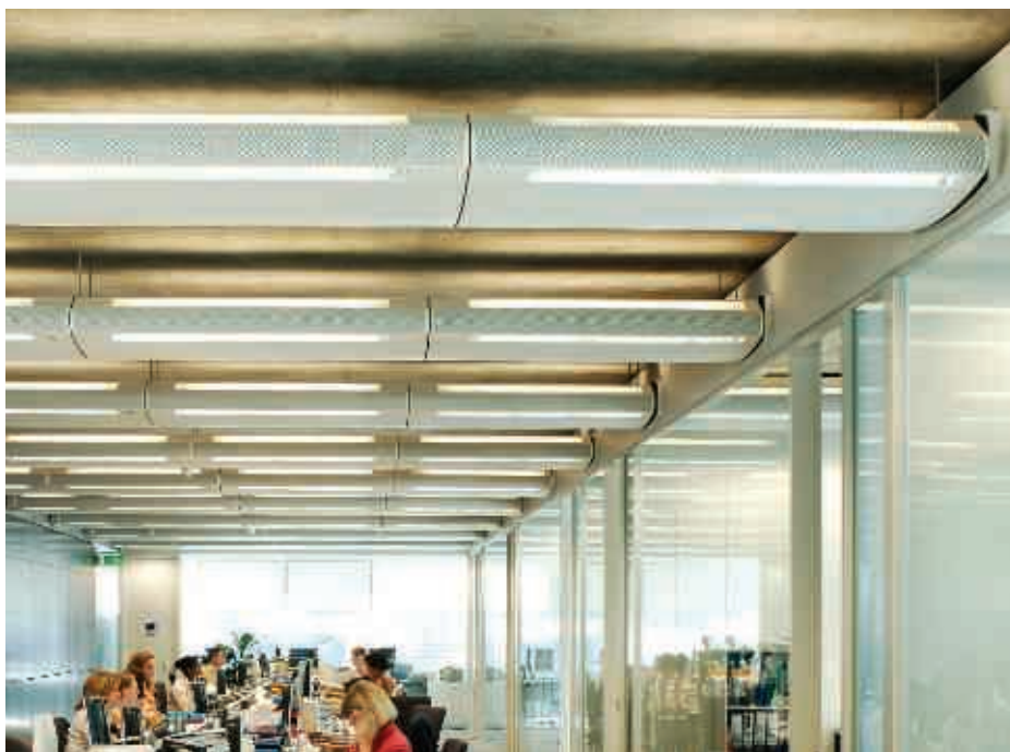
Integrated service modules from SAS are space saving and deliver air-conditioning more efficiently than fan-coil systems. This installation is at Imperial College in London.
